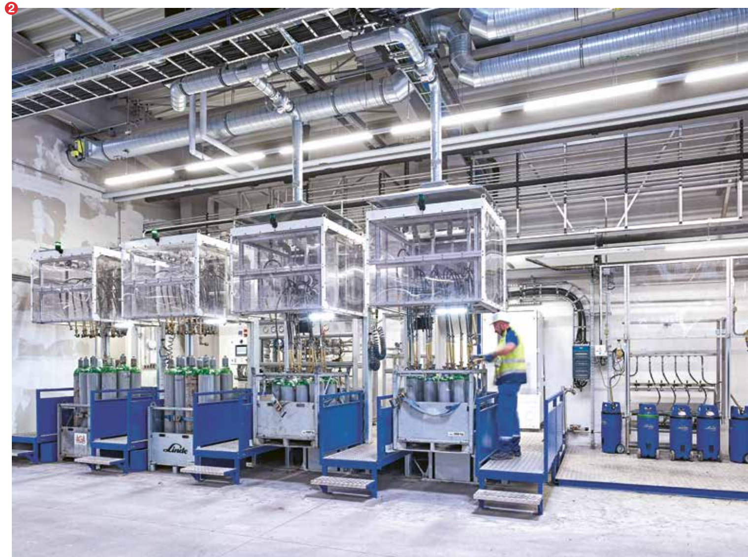
2 Project: Linde Gas, Marl, Germany Product: Modario® trunking system
